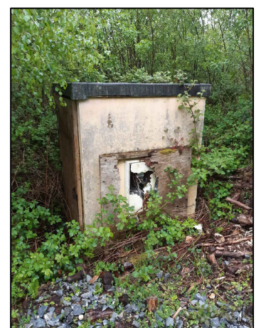
Existing ESB Kiosk to be Decommissioned and Demolished
